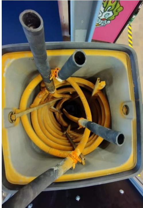
Figure 37: Plastic coil inside solar boiler.
