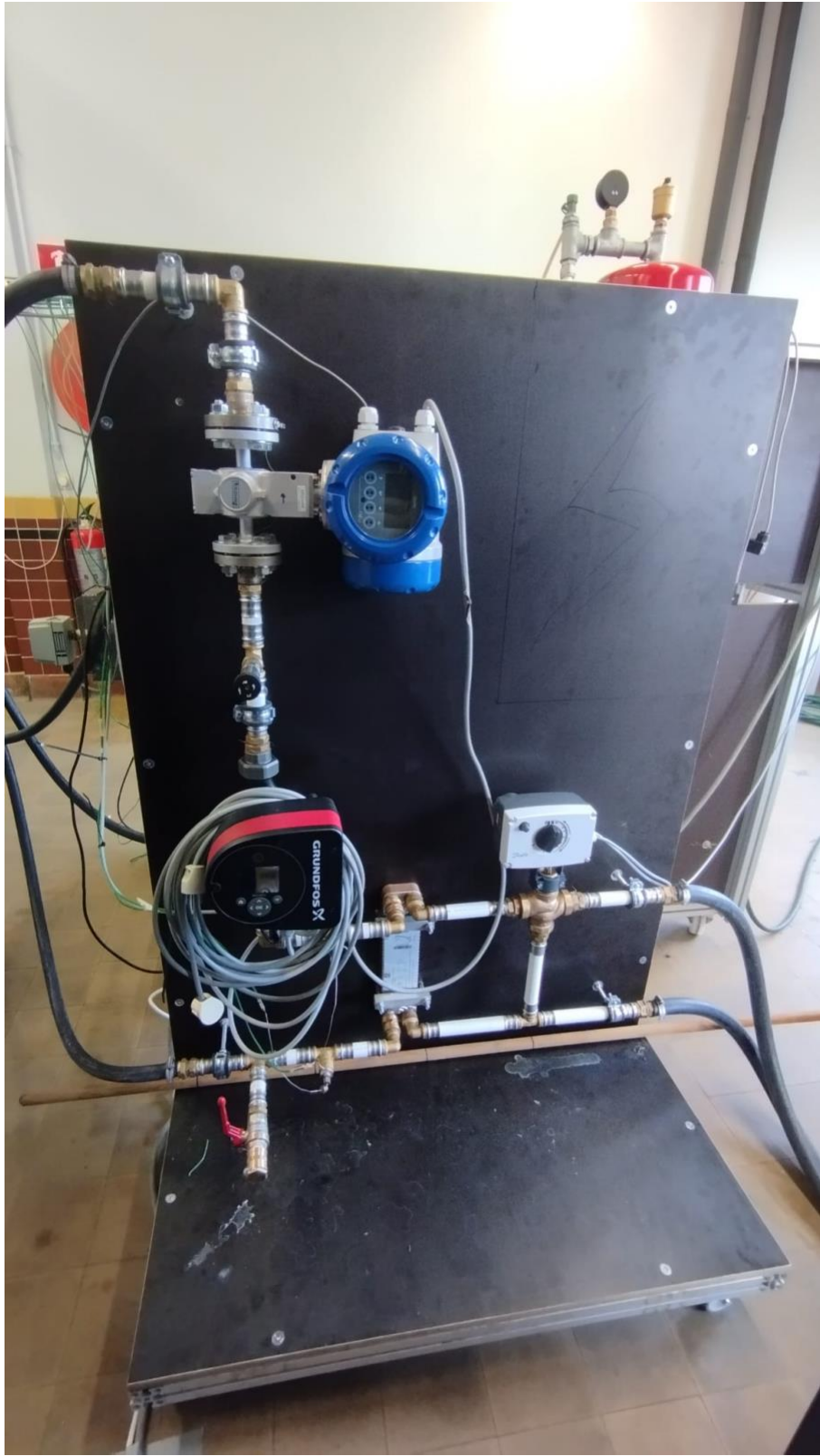
Appendix C: Photo of cold circuit and chiller circuit.
