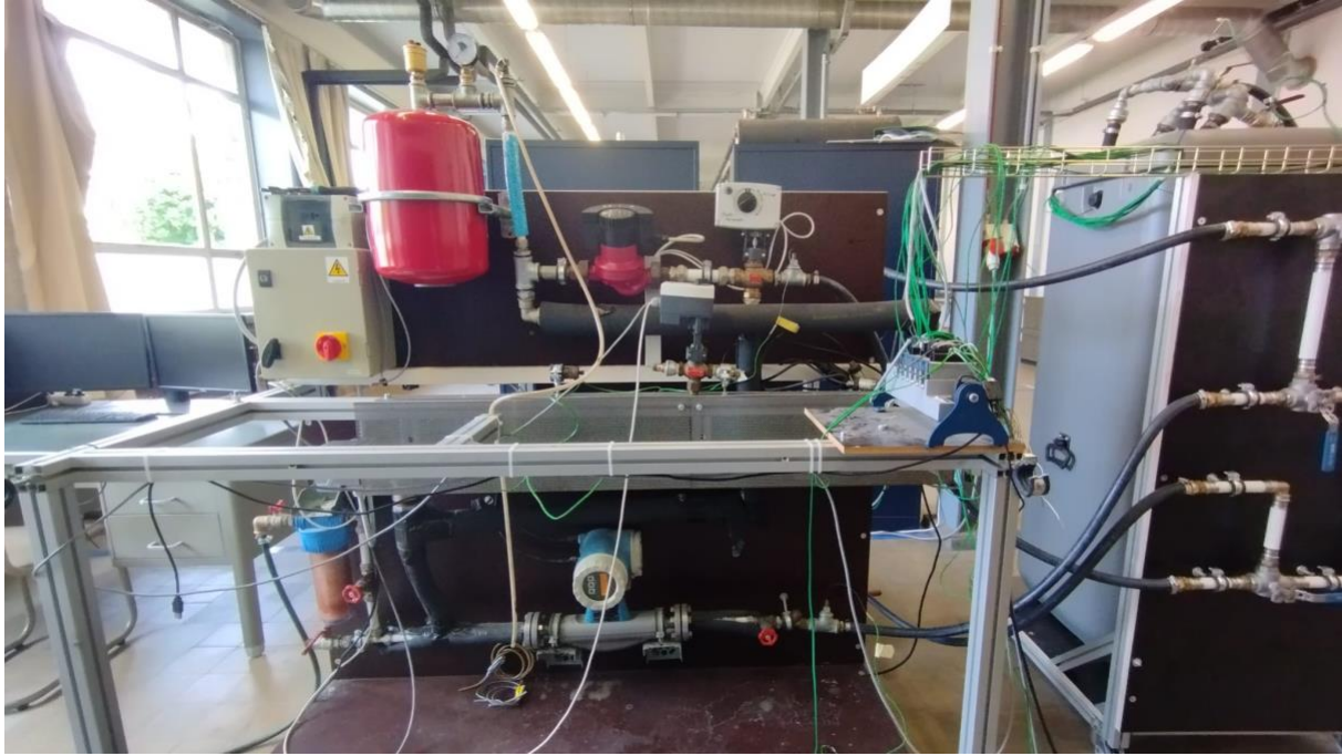
Appendix A: Photo of hot circuit.
