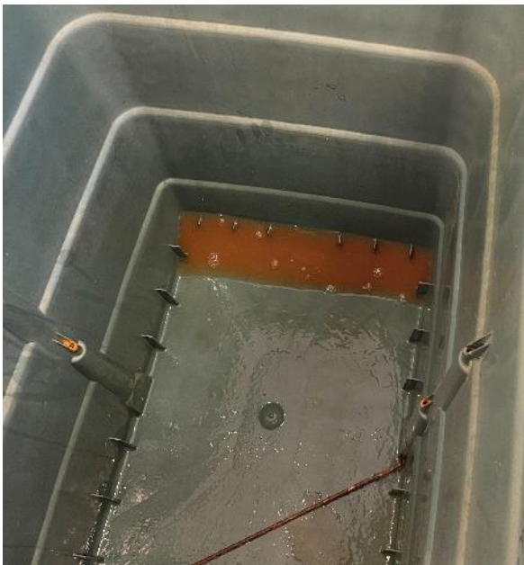
Figure 4-10: Red sludge present in the filtration system
