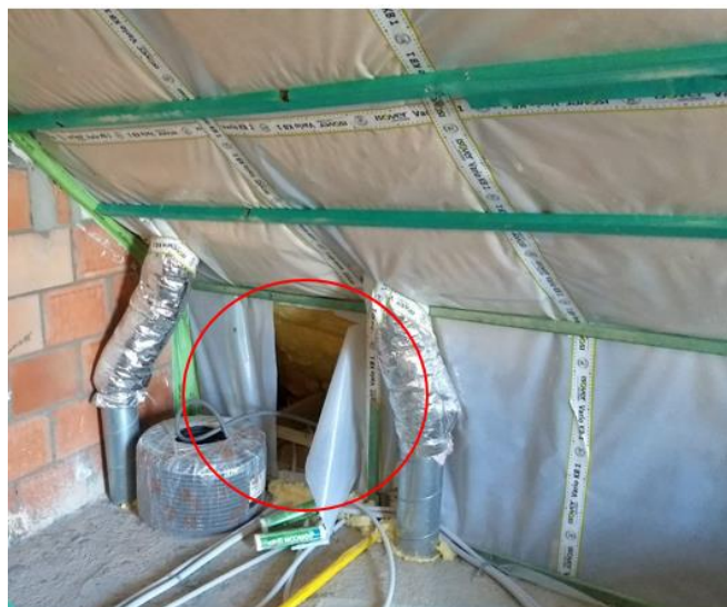
Figure 21: Bad execution of the vapour barrier
