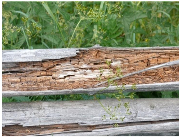
Figure 11: Cubic fracture pattern after brown-rot decay [10]
