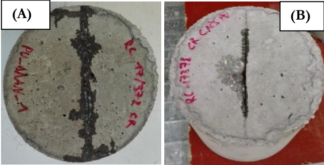
FIGURE 8.3: DIFFERENCE IN LEAKAGE OF THE HEALING AGENT AND SPALLING OF THE CONCRETE BETWEEN SPECIMENS WITH (A) MANUALLY INJECTED CRACKS AND (B) EMBEDDED CAPSULES
