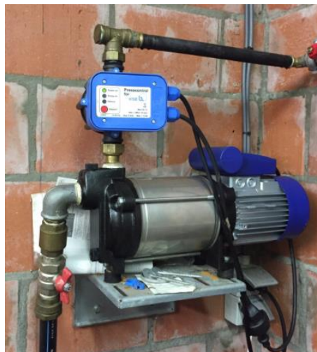
Fig. 2.16: Pump of rainwater treatment system
