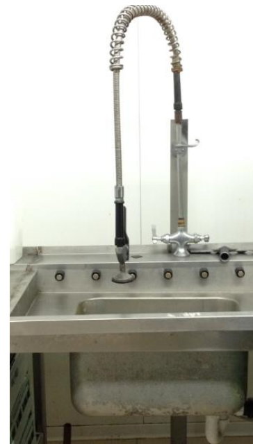
Fig. 2.15: Pre-rinse spray supplied by rainwater
