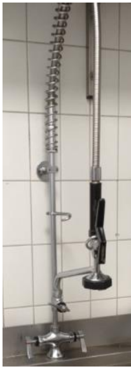
Fig. 2.11: Pre-rinse spray used in the kitchen
