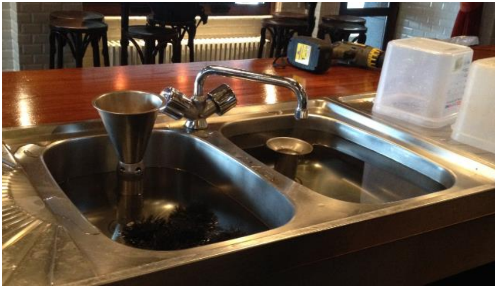
Fig. 2.8: Double compartment sink located in the bar
